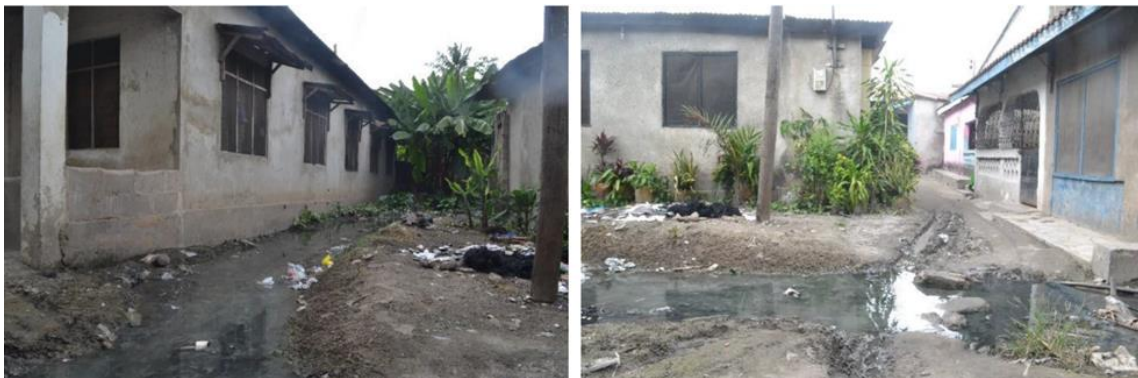
Figure 6: Photos showing an example of the water from bathrooms discharged to alleyways and affecting the front verandas as space that were used collectively by the residents. Source: Fieldwork (2023).
