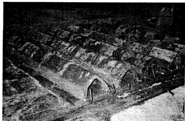
Plate 3: Plastered and hardened slab strips, lifted and arranged to form a slab panel
