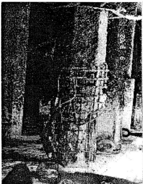
Plate 3: Exposed reinforcement in one of the piers at main quay
