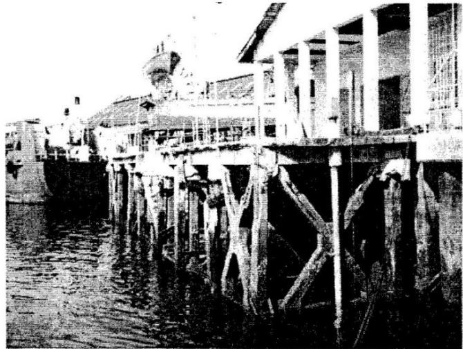
Plate 1: Concrete piers and struts severely corroded at Lighter quay .
