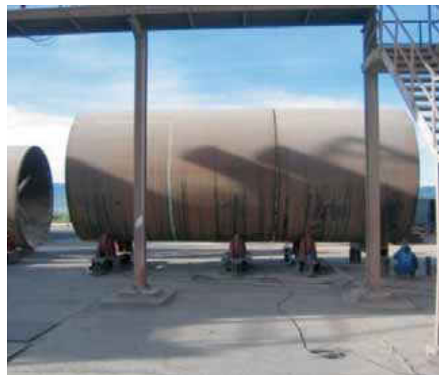
Fig. 12: New segments of kiln shell being welded on the ground before being hoisted into position.
