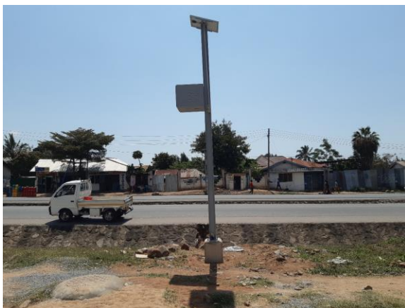
Figure 5: Inductor loop control box installed along the road in Mwanza region.
